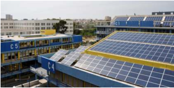
View on the roofs of the faculty with solar panels. (Photo: https://cssc11.campus.ciencias.ulisboa.pt )
